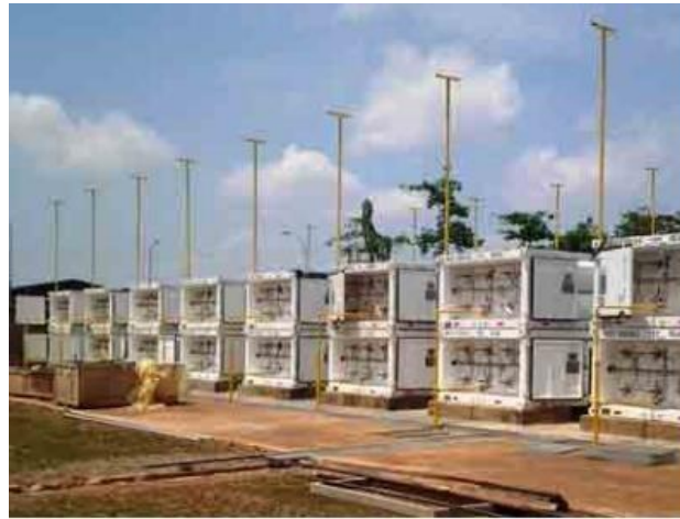
Figure 2.1 CNG Mother Station Jakabaring (Gas and Fuel Division of PT. PLN Persero, 2013)
